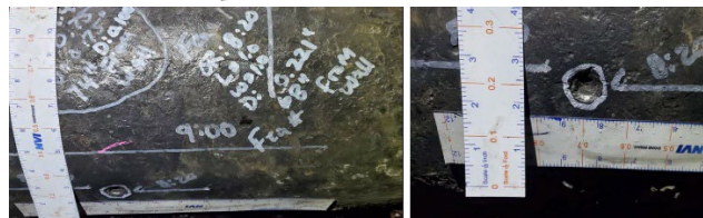
Deep metal loss of 88.4%
